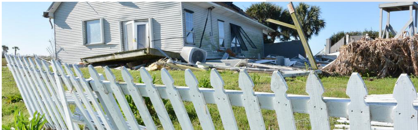
The effects of a tornado on a residential property in Madisonville, Louisiana. Property damage presents a significant challenge for survivors of catastrophic disasters. Source: Sharon Karr
