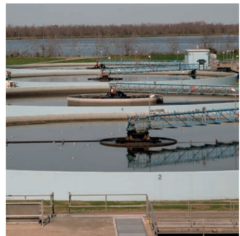
FEMA has obligated more than $89 million in funding for repairs to New Orleans Sewerage and Water Board’s Eastbank Sewerage treatment facility. Image: Manuel Broussard/FEMA
