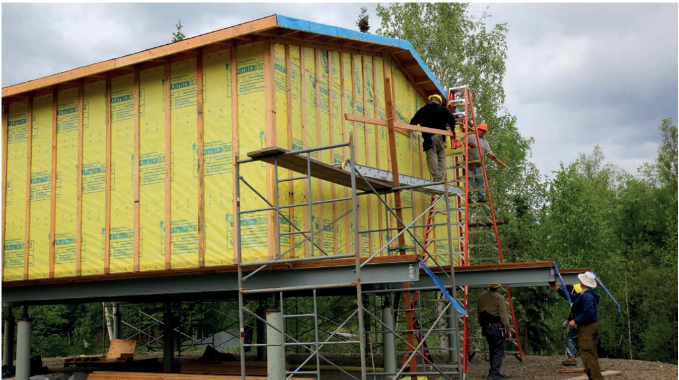
Volunteers from Samaritans Purse and United Methodist Volunteers work together to build a Cold Climate Home for a disaster Survivor in Galena, Alaska. Image: Adam DuBrowa/FEMA
