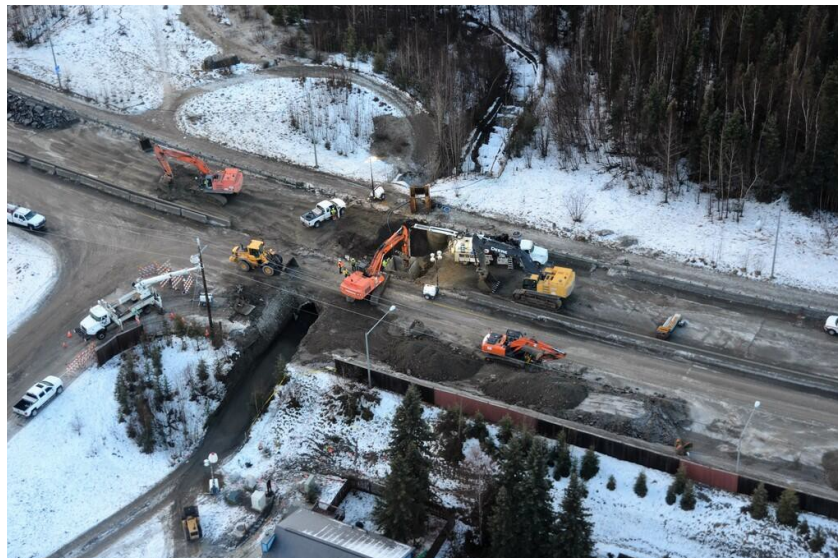
The type of coordination described above can be employed to expedite a variety of disaster recovery infrastructure projects, like the repair of this road in Alaska after the November 2018 Alaska Earthquake (Credit: FEMA/ Savannah Brehmer)
